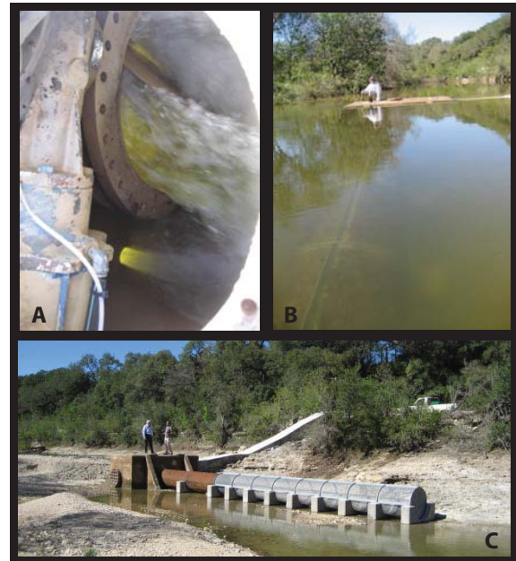
Figure 3. A) Water entering the intake system; B) Water level almost above vault; C) Upgraded intake system during low flow.
